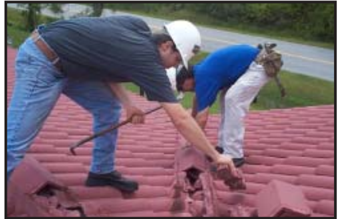
Tim Williams and Brad Guy of University of Florida Center for Construction and Environment deconstructing barrel tile roof of Veterans Highway house (7/02)
